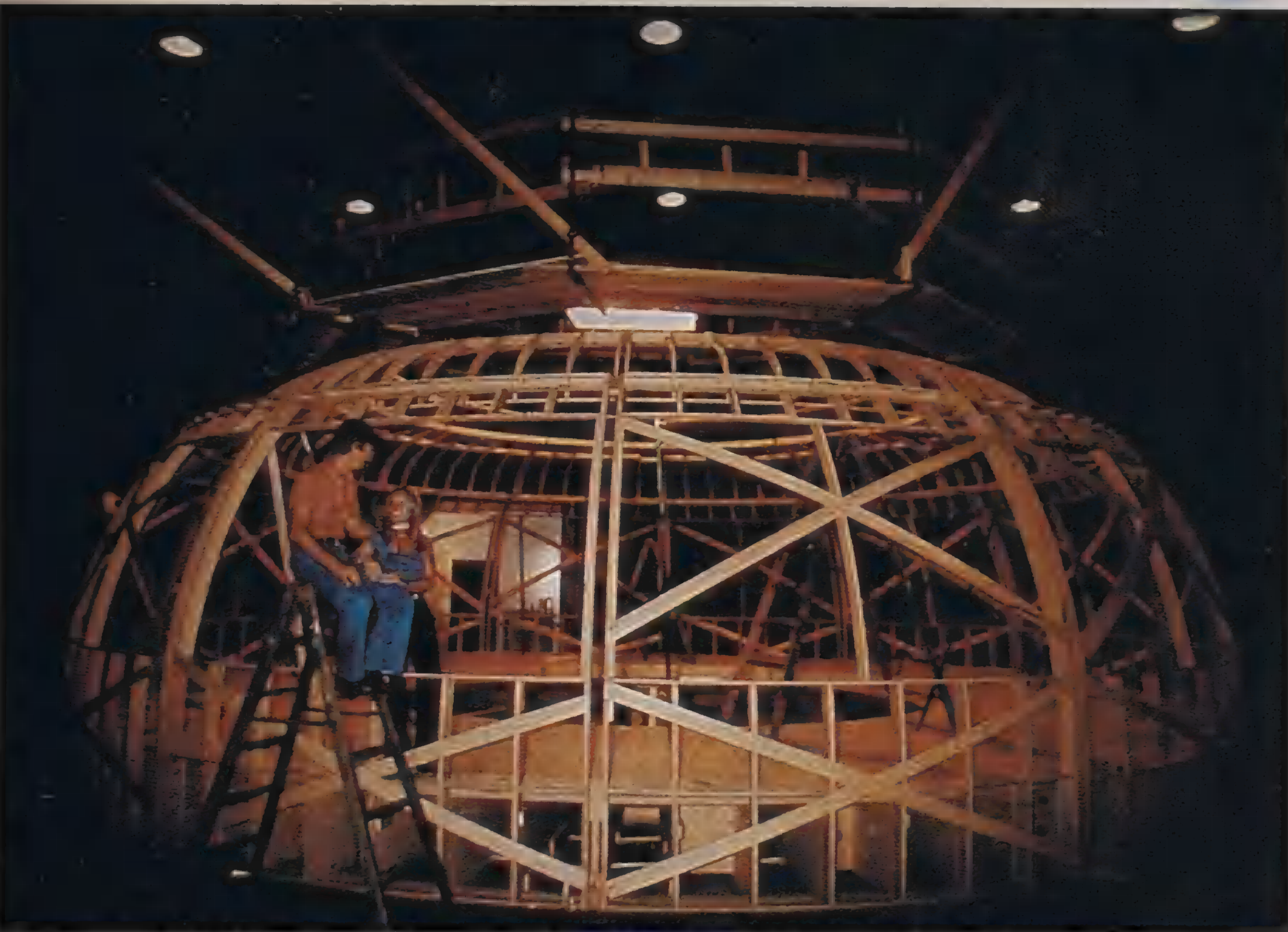
The Enterprise bridge set under construction. All of the walls have been made "wild" — each one can be removed to allow for filming from a variety of angles.
